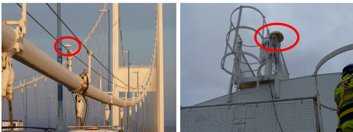
Figure 4. The illustrations of bridge cable surveying point antenna installation (left panel) and tower surveying point antenna installation (right panel).
